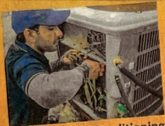
Heating & Air Conditioning
