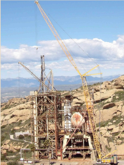
Coca Test Stand I is at the center of NASA's Phase 7 demolition.
