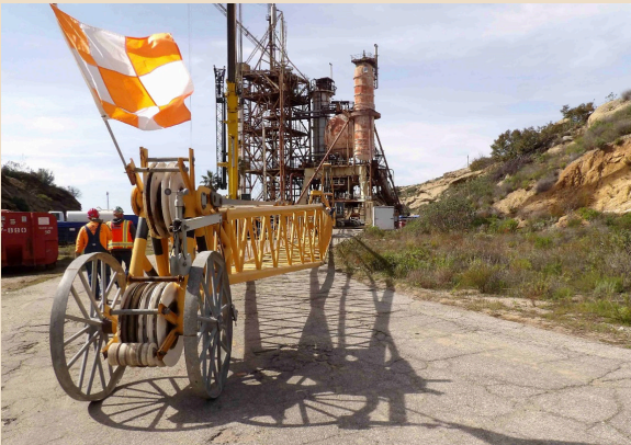
Demolition crews attach the boom (the telescopic arm used to lift heavy objects) to the crane.
