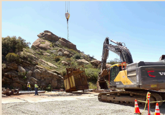
Workers look on as a crane moves an elevator car that was once used to transport workers to different levels of the test stand during historic operations.
