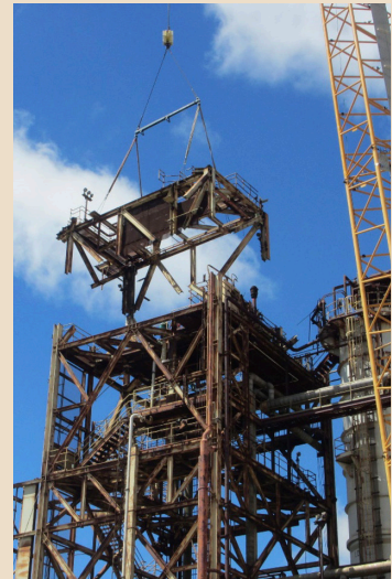
Above: A 300-ton crane removes Level 7 of the Coca Test Stand I during demolition.
