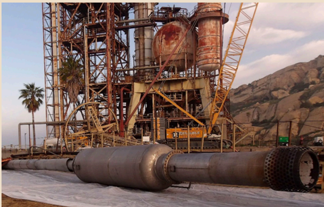
The flame stack that stood atop Coca Test Stand I sits in front of the structure following its removal.
